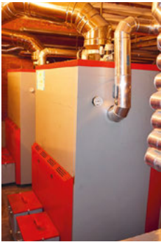
Fig. 5.74: Biomass pellet boiler in Colegiata de San Isidoro, León, Spain
