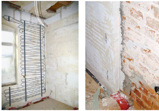
Fig. 6.7: Wilhelminian building, wall-heating surface, application of iQ-Therm insulation system to the outer wall
