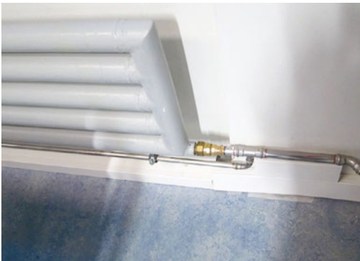
Fig. 9.4: CS5, Original radiator with new pipes inside the thermal envelope
