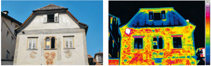
Fig. 1.4: IR-thermography of the south facade shows homogeneous brickwork in natural stones and material change at the exterior top floor wall.
