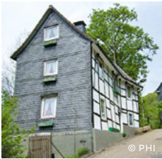
Fig. 2.8: Slates as protection against driving rain on the windward side of a traditional German half-timbered house
