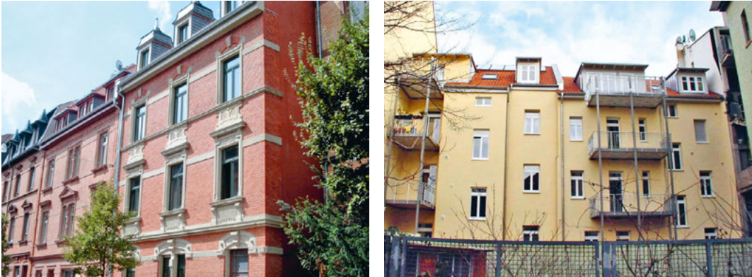
Fig. 4.10: Historic town house after renovation with interior insulation on the street facade and exterior insulation on the rear facade (amongst other measures). The heating demand could be lowered by approx. 80 % while preserving the appearance of the building.
