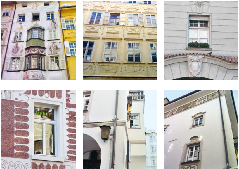
Fig. 1.15: Originally, the wooden frames, impost, and sash bars were very fragile and thin, possibly moulded (a-b-c), while the appearance of the typical replacements is much broader (simple application of the IV68 standard, d-e-f).
