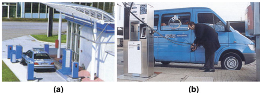
Fig. 3.29 Liquid (a) and gaseous (b) hydrogen distribution unit
