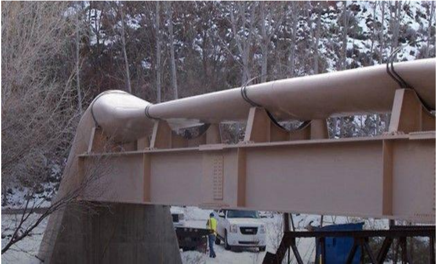
DOWN-SURGE INDUCED Pipe Collapse
