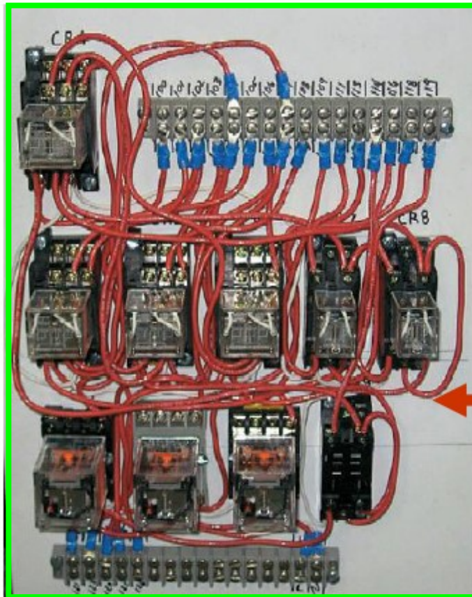
Relay control panel
