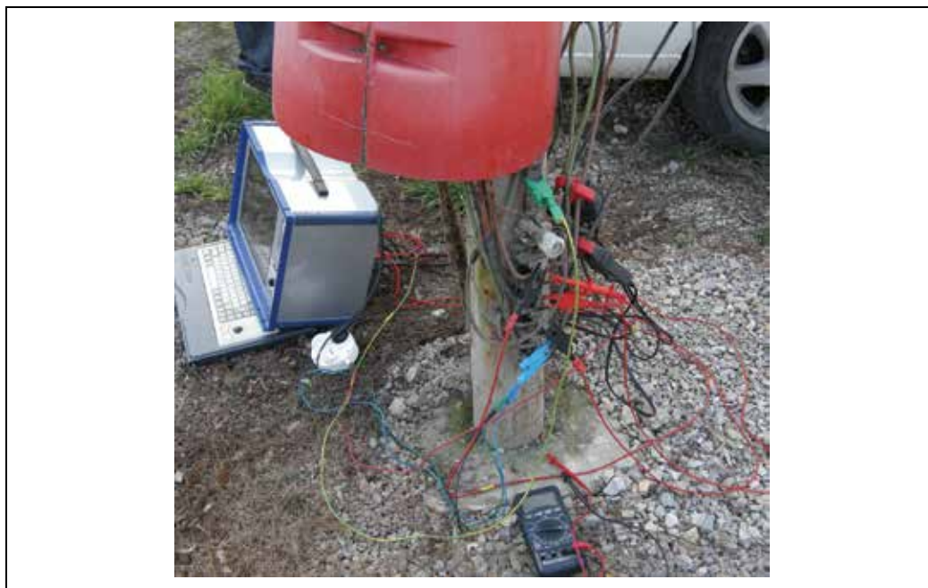
Fig. 15. Measuring power quality in public lighting network
