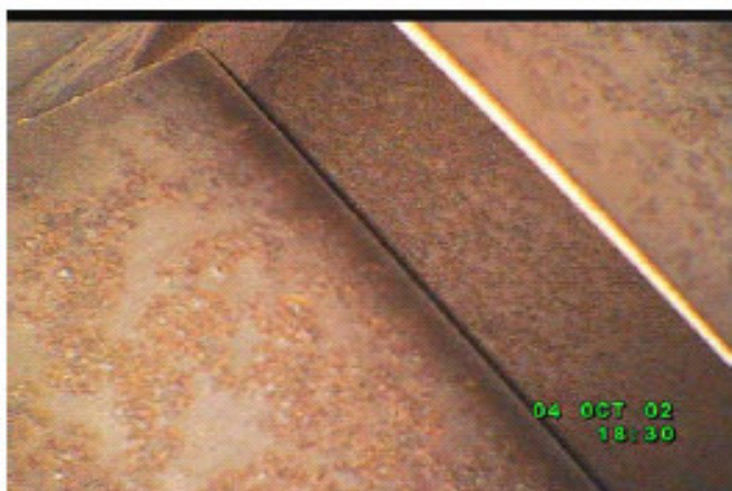
Corrosive deposits on 13 th stage Compressor Rotor blades & Stator vanes.
