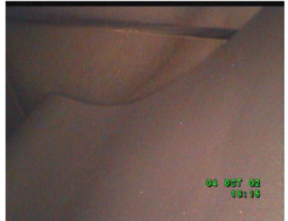
A view of stage # 2 variable Nozzle root, leading edge & Pr side.
