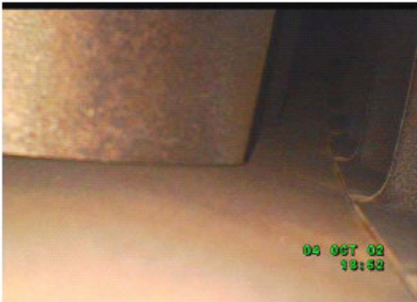
Compressor Rotor blade tip in satisfactory condition
