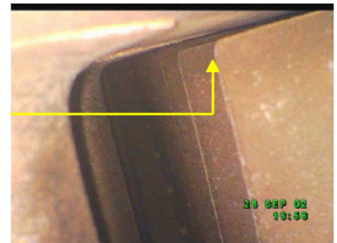
Trailing edge thinning noticed on Stator vanes.
