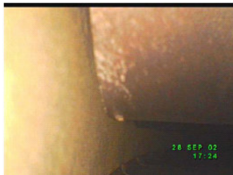
Trailing edge thinning & rounding noticed on Rotor Blades.
