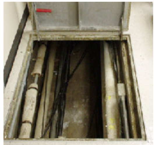
Live steam lines? Electrical lines?
