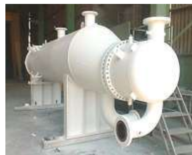
Heat Exchanger Final Painting Evaluation
