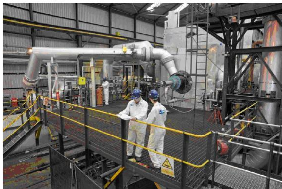
Fig. 4 40 MW test burner facility at Doosan Babcock's Renfrew facility. Image copyright of Doosan Babcock Energy Limited
