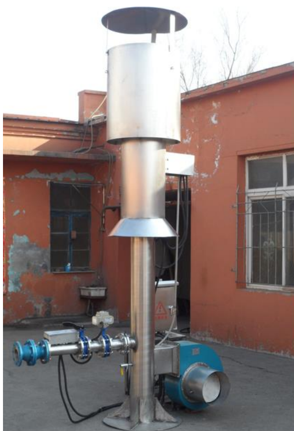
Figure 9 An enclosed flare from CAMDA.
