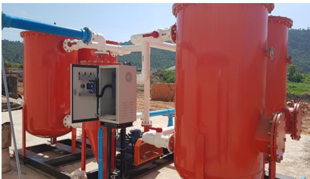
Figure 7 Biogas pre-treatment unit at M's Pig farm.
