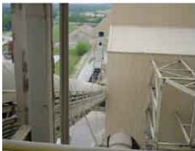
Conveyors to Kiln
