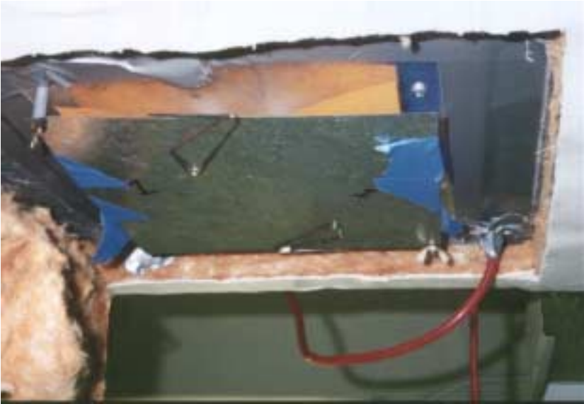
Figure 6. Impaction plate installed in Building LS-2
