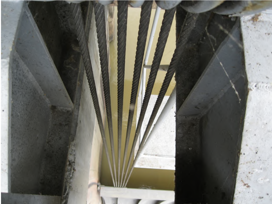
Figure 16-4. Wire Ropes for Lifting a Tainter Gate.
