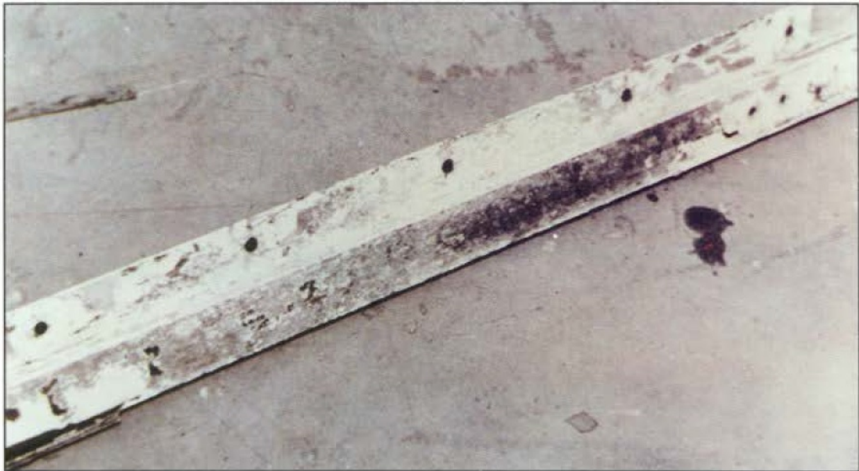
Figure 2-3. Uniform Etch Corrosion
