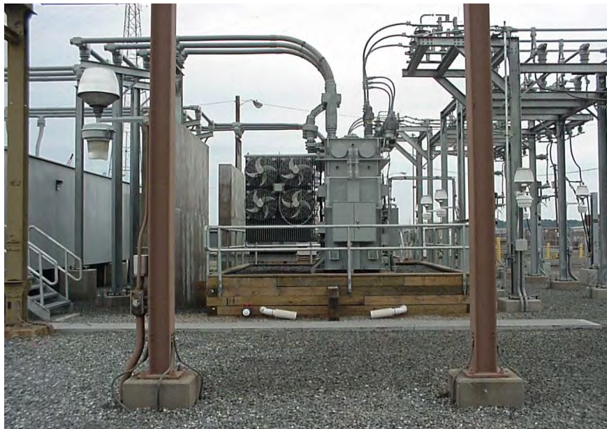
Figure 5 - New 13/4 kV Transformers and 13 kV Switchyard
