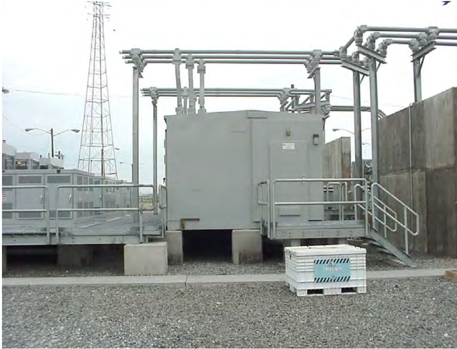
Figure 6 - Metal Enclosed 4 kV Switchgear [Outside View]
