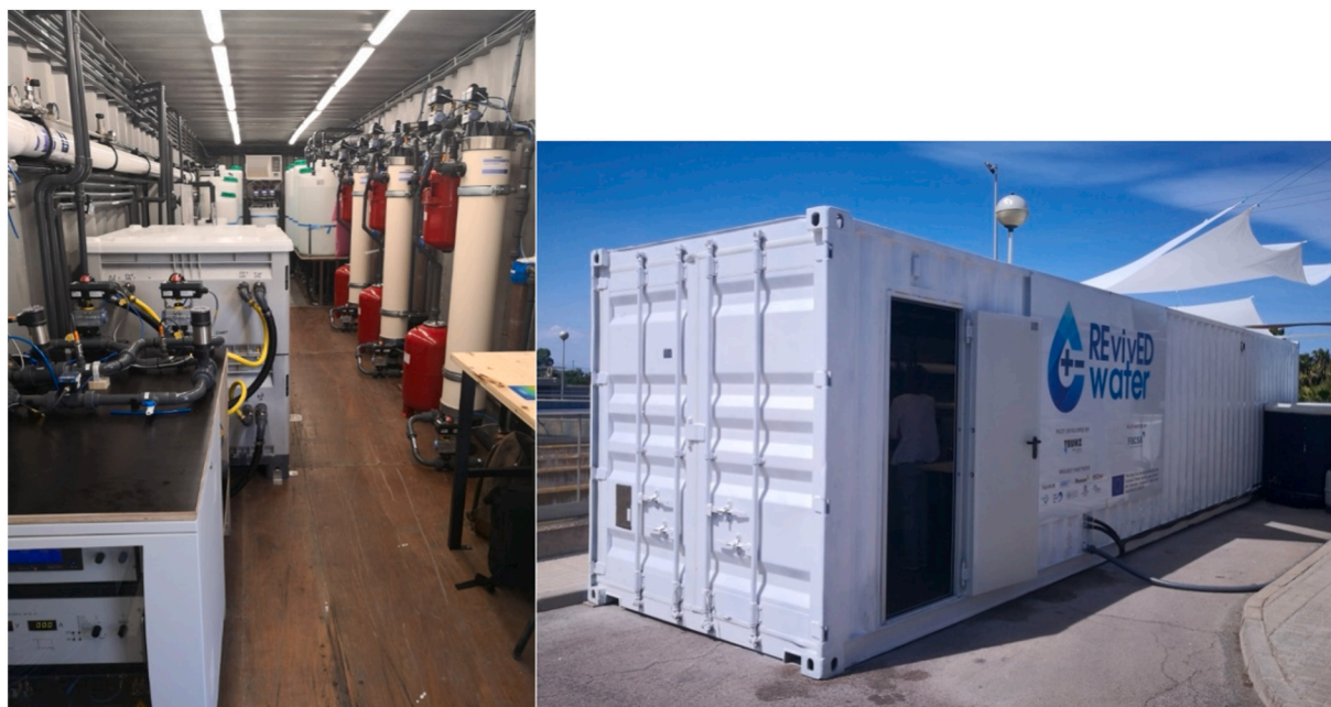
Fig. 2. Picture of the integrated EM process-RO pilot plant (left) installed in a container (right) at the FACSA WWTP in Burriana, Spain.
