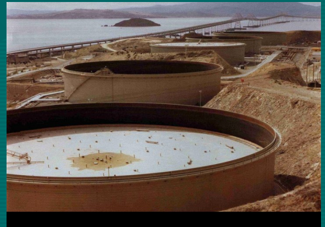
Floating roof tank
