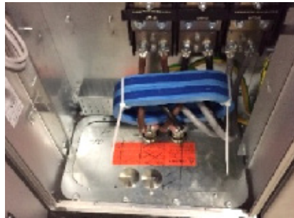
Fig. 6.21 Common-mode cores installed at the drive terminals
