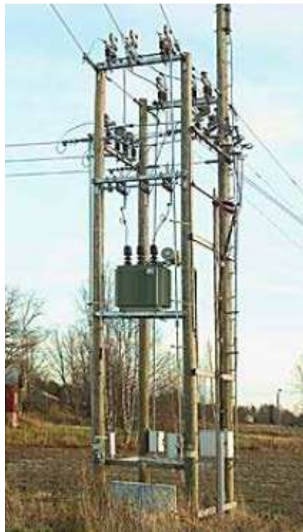
Figure 3.119: Pole-mounted secondary distribution substation
