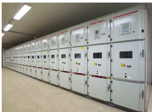
Figure 3.47: Air-insulated primary switchgear equipped with Feeder Terminals
