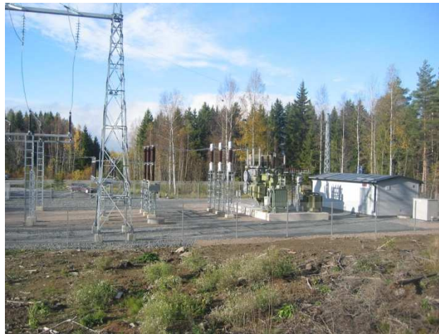
Figure 3.2: A typical rural primary distribution substation 110/20kV
