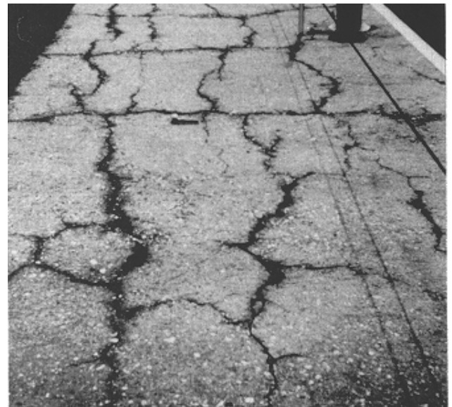
Figure 2-6. Pattern cracking resulting from alkali-silica reaction
