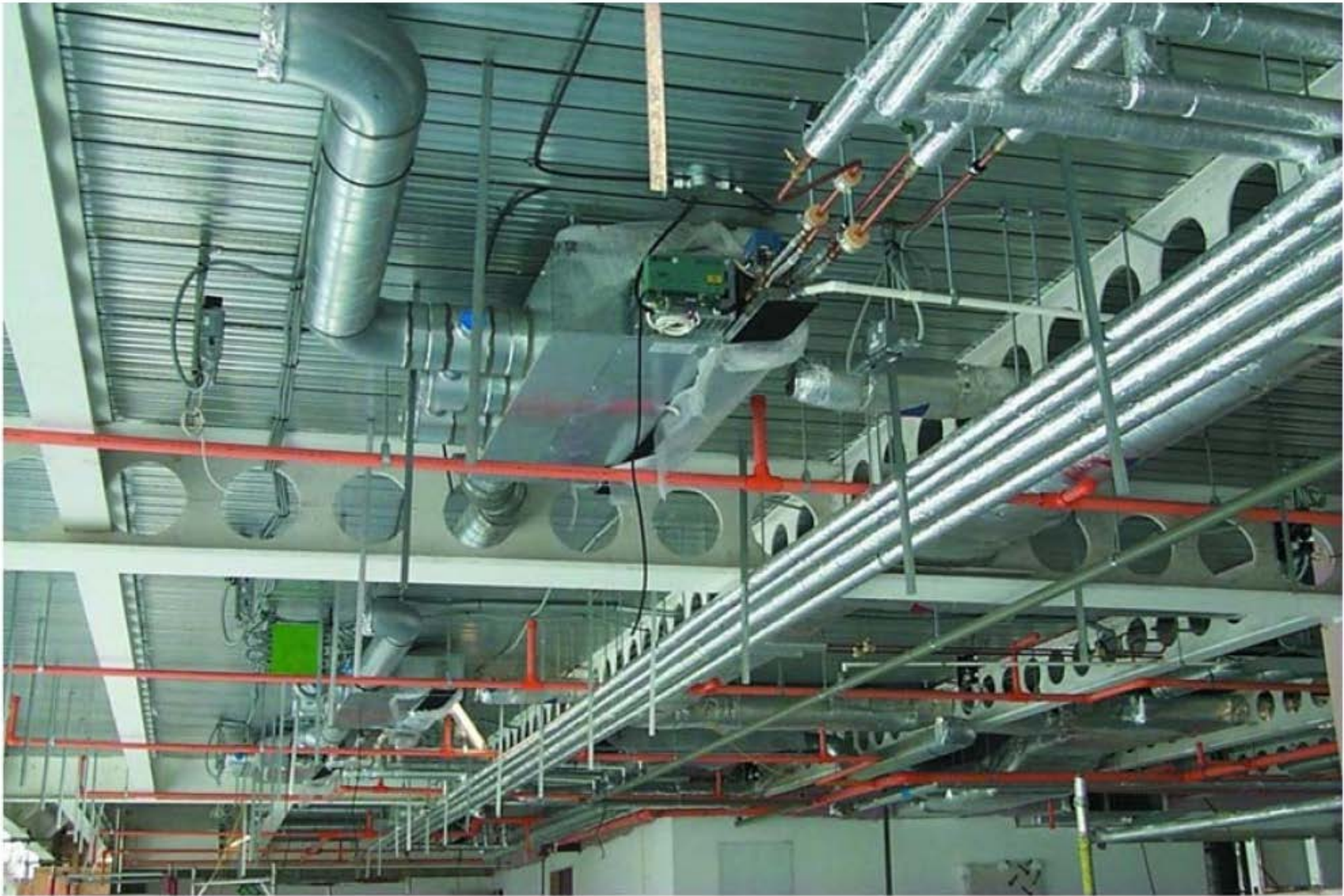
Coordination between ductwork and structural element
