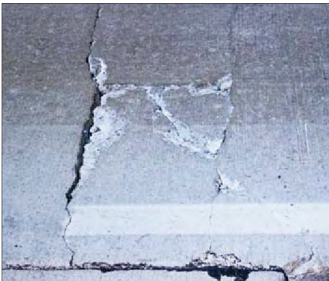
Figure 7. A typical CRCP punchout distress.
