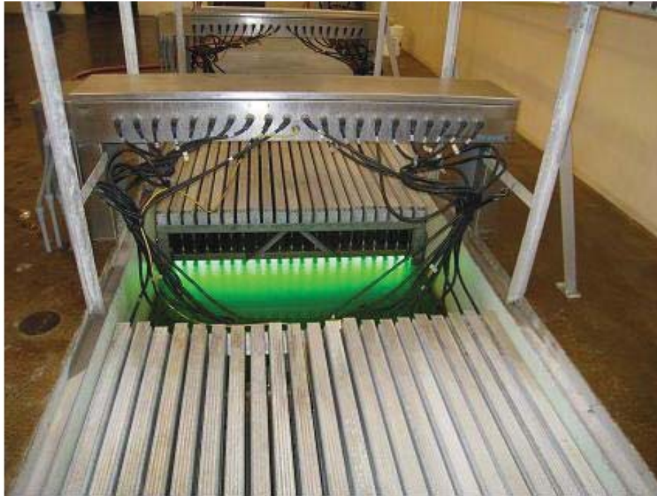
Photo of Sparta Wastewater Treatment Plant
