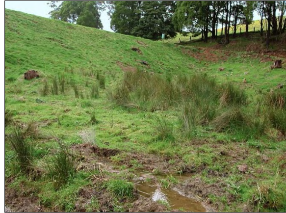
Earthen dam seepage
