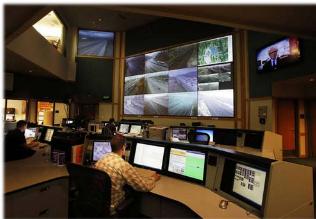
Figure 9. Photo. Traffic Operations Center. (Source: Utah Traffic Operations Center)
