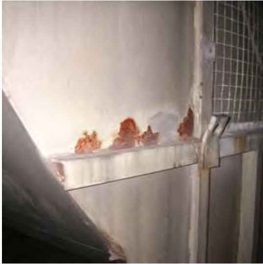
Figure 4.54 – Corroded fan housing.
