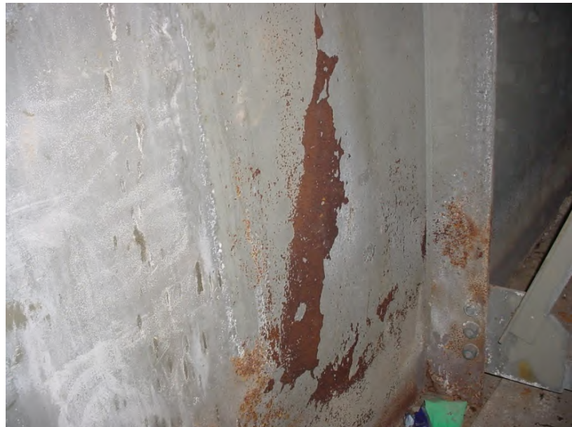
Figure 4.13 – Minor corrosion along roof girder.
