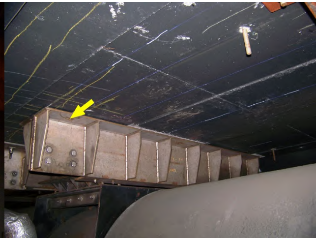
Figure 4.44 – Missing bolt at longitudinal fan support.
