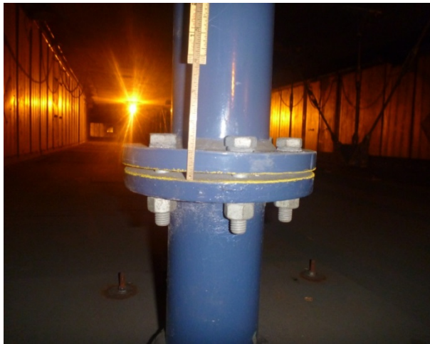
Figure 4.43 – Sign support with gaps at connection.
