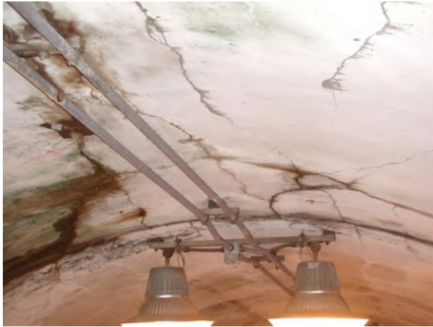
Figure 4.21 – Cracks with rust stains.
