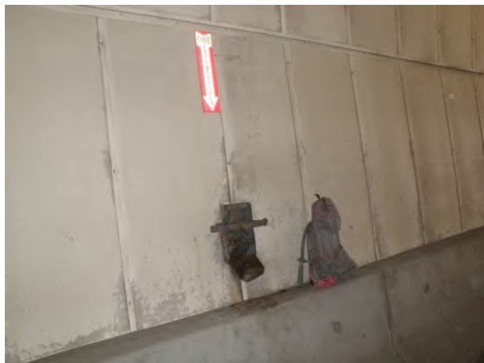
Figure 4.72 – Missing fire extinguisher.
