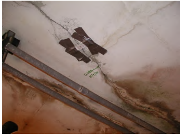
Figure 4.22 – Medium width crack in concrete liner.
