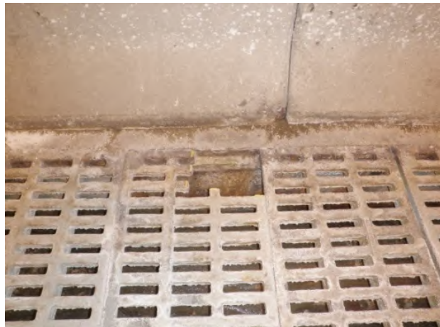
Figure 4.58 – Broken scupper grate.
