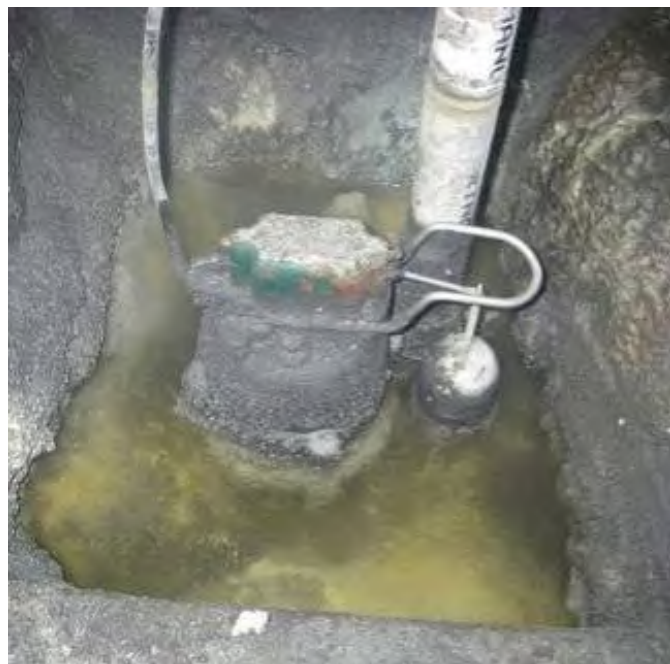
Figure 4.61 – Accumulation of calcium deposits at sump pump.
