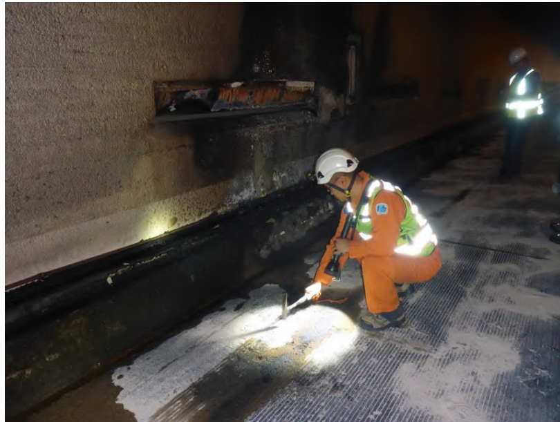
Figure 4.6 – Evaluating fire damage.
