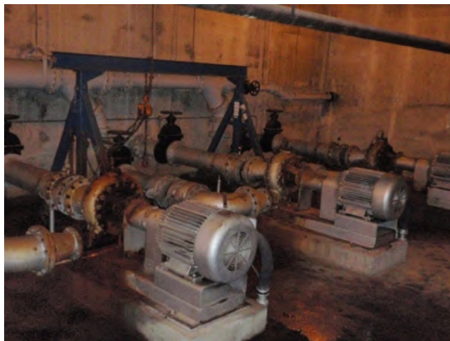
Figure 4.59 – View inside pump room.
