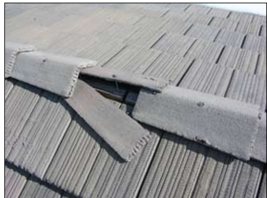
Figure 3. Displaced tiles allow ember entry.
