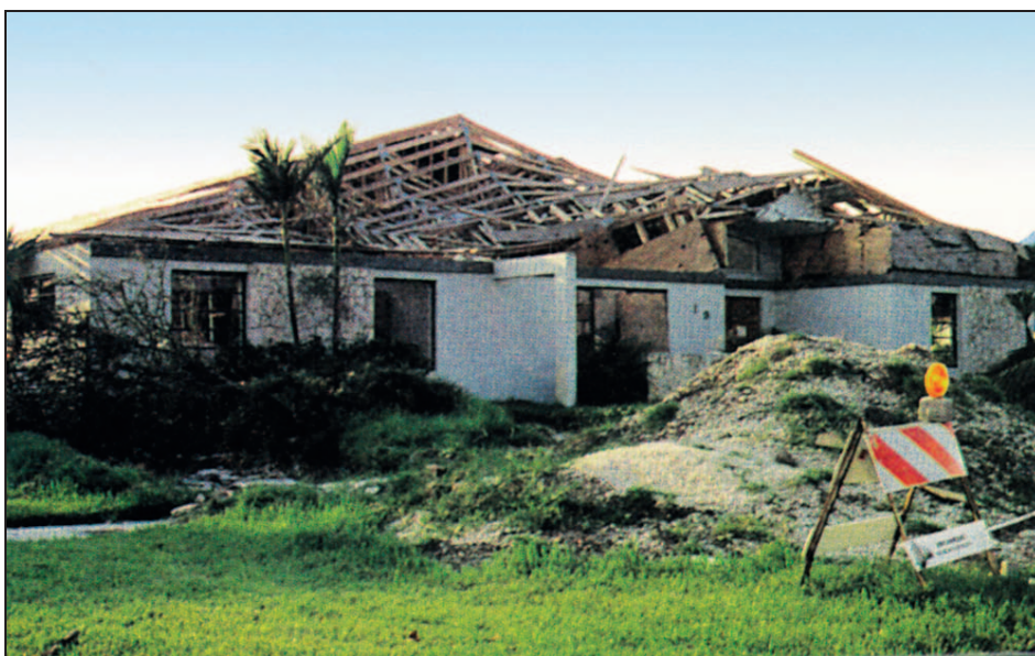
Figure 9-21. Gable-end failure, Hurricane Andrew (Dade County, FL, 1992)
