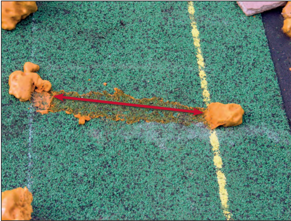
Figure 11-44. Adhesive that debonded from the cap sheet
