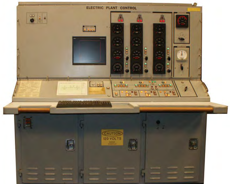
Figure 6-28 — Electrical plant control console.
