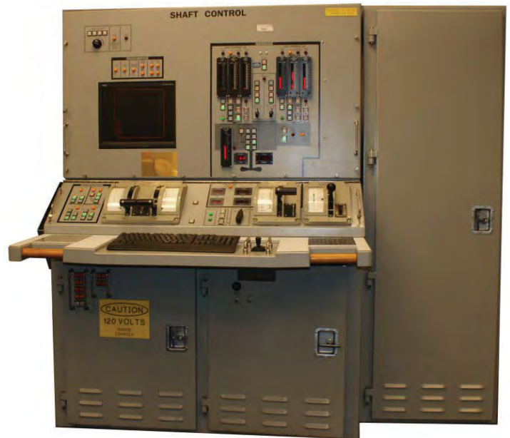
Figure 6-30 — Shaft control unit.
