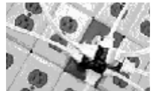
Overloads are a major cause of fires.
