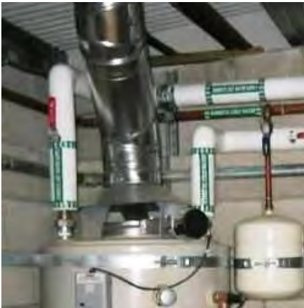
Figure 32. Stainless steel flue on storage heater.
