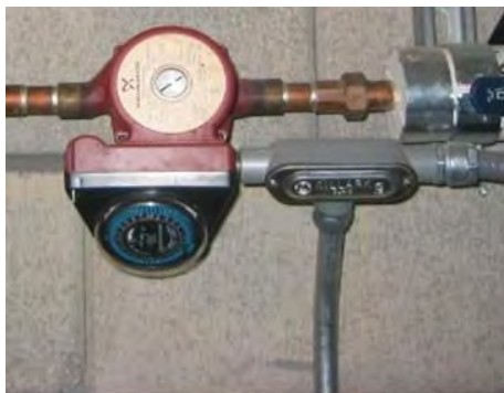
Figure 10. Timer mounted on a recirculation pump.
