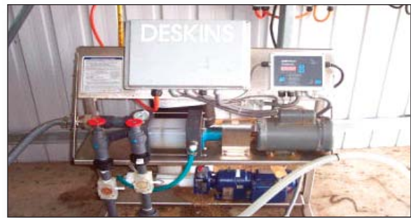
Polymer Preparation Unit
