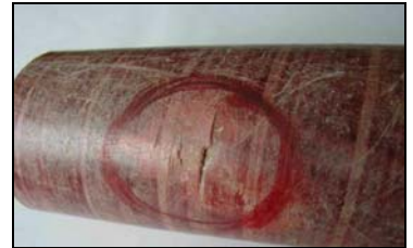
Fiberglass piping is cracked
