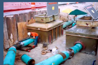
Hydrant piping vaults
