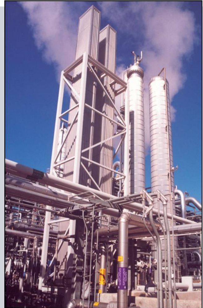
BASF, Port Arthur, Texas
