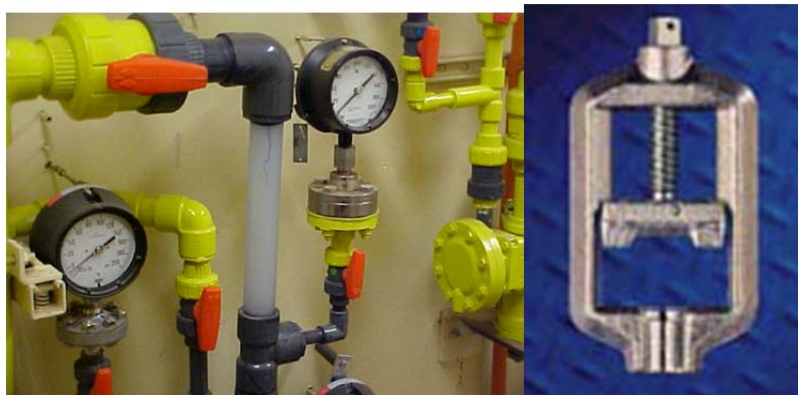
Chlorine piping and chlorine cylinder yoke.
