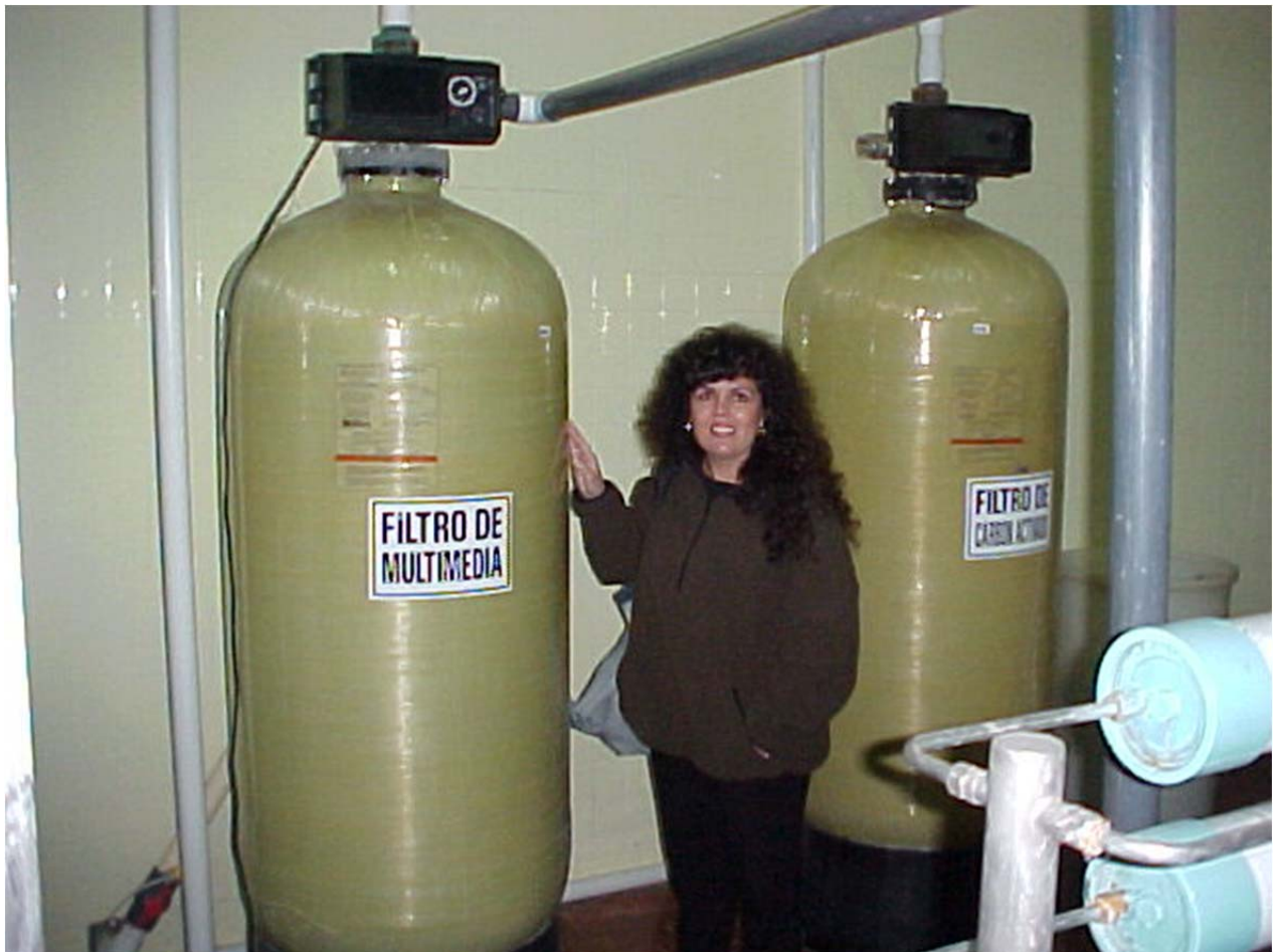
Commonly found packaged filter system components.
