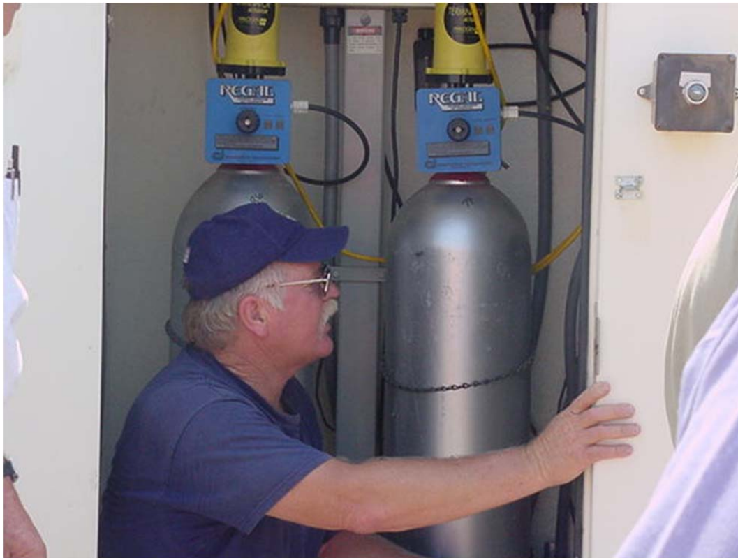
150-pound Chlorine Cylinder
