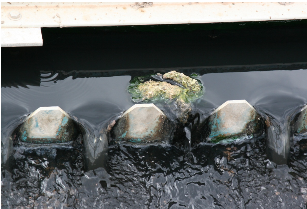
Caked grease stuck on weir.
