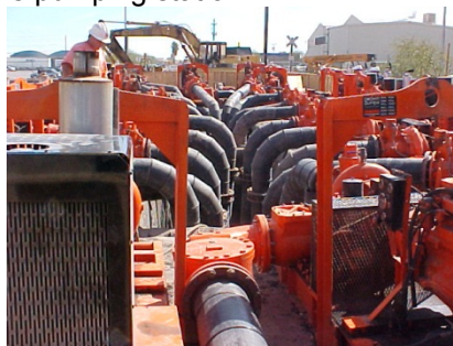
Pumps at a temporary sewer manhole by-pass.
