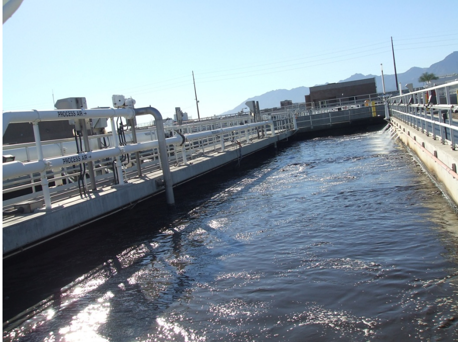
Anoxic zone, denitrification area.
