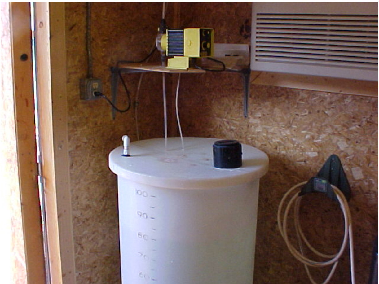
Small Chlorine solution tank.
