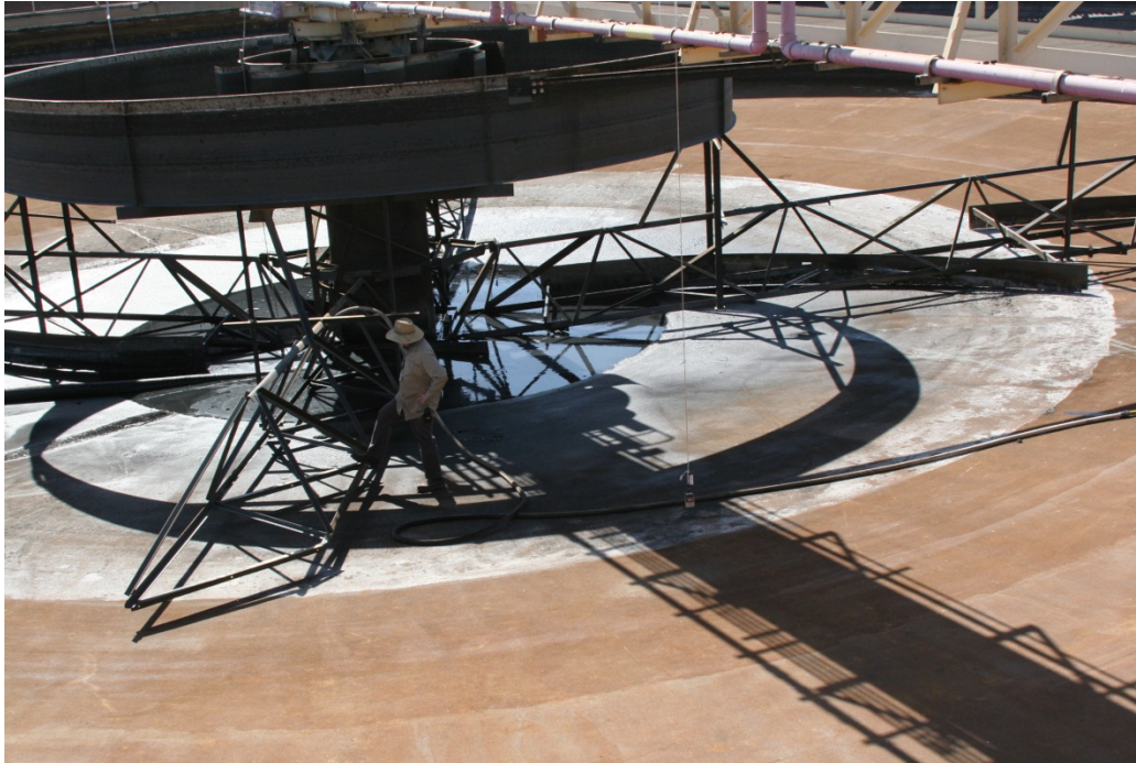
Scraping mechanism inside a clarifier.
