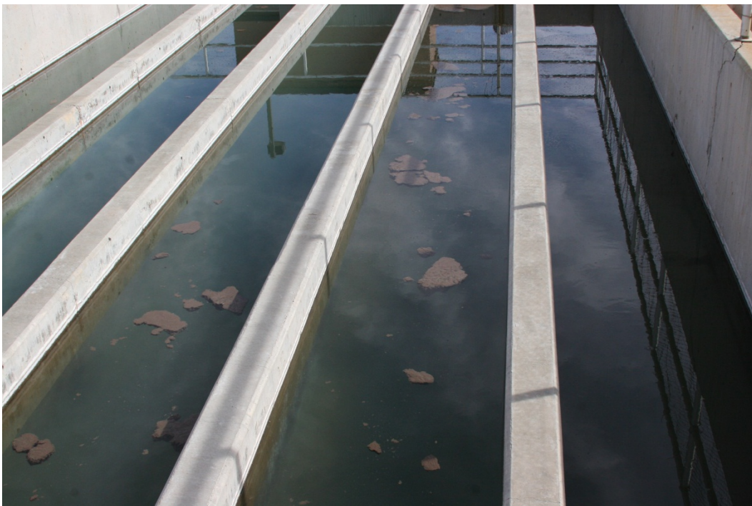
During a plant upset, sludge from the filters can be carried over to the chlorine contact channel. In this photograph, it is not too bad, I've seen much worse.
