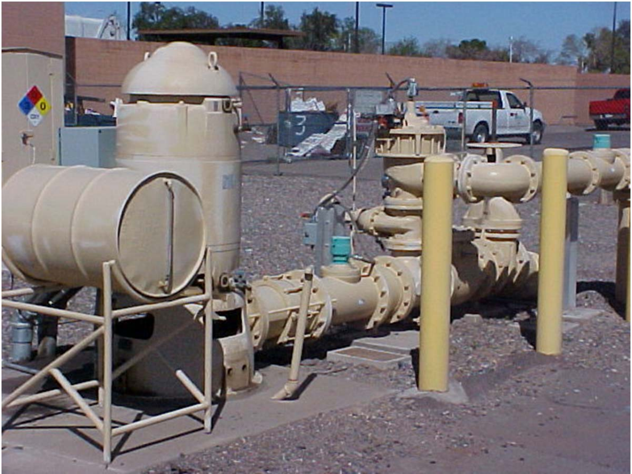
Groundwater production well with a mineral oil sealed vertical turbine pump. Sometimes, this mineral oil will get into the distribution system.
