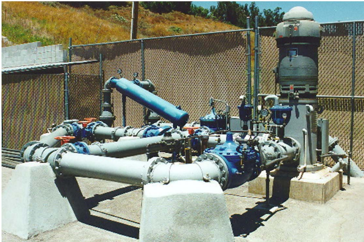
Vertical Turbine Well
