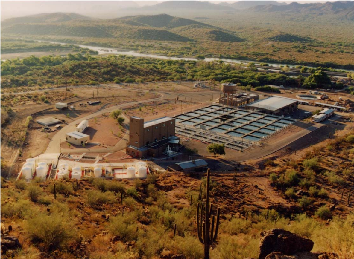
Here is a surface water conventional treatment facility next to a river.
