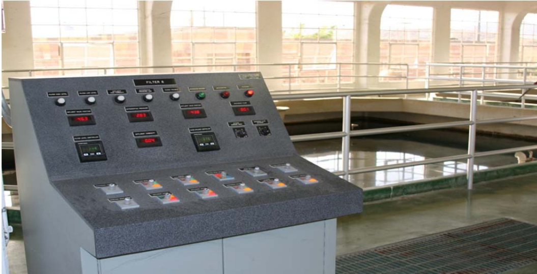
This is a filter control panel.
