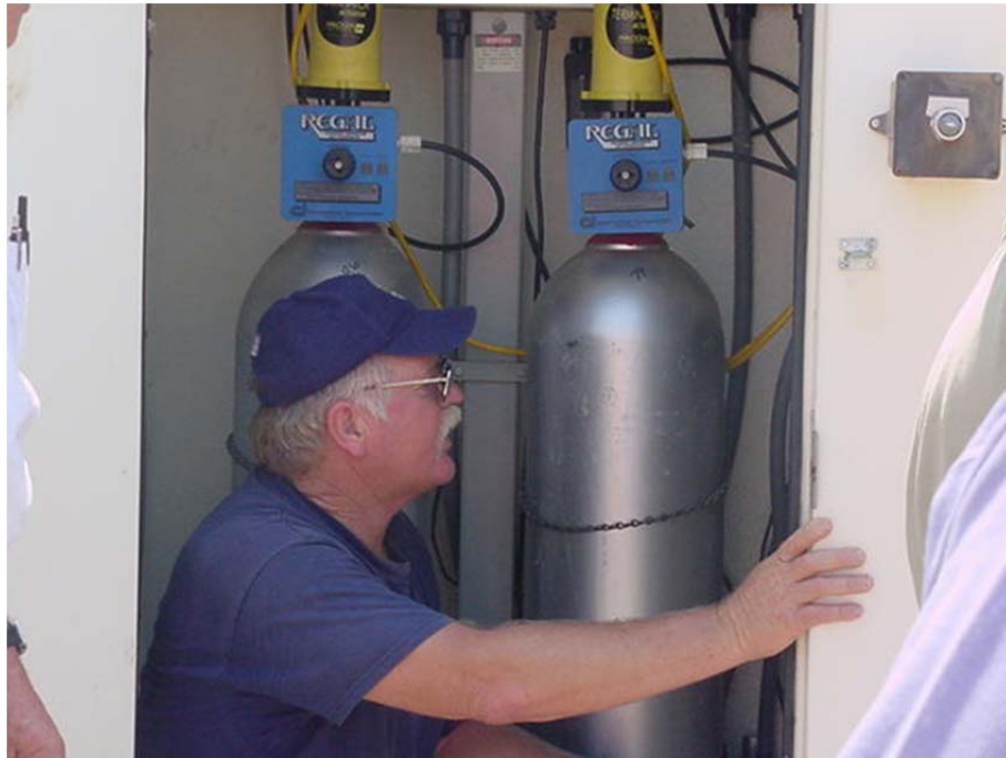
150-pound chlorine gas cylinder.
