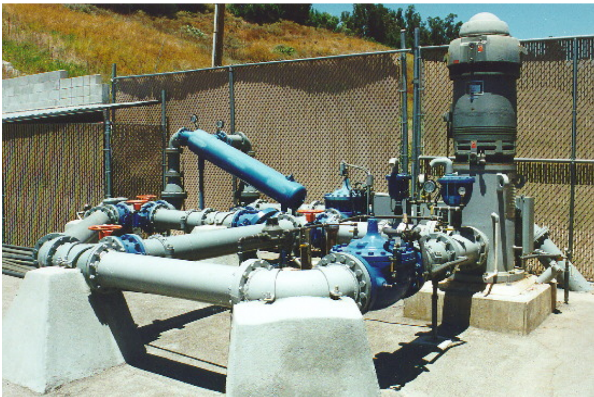
Vertical Turbine Well
