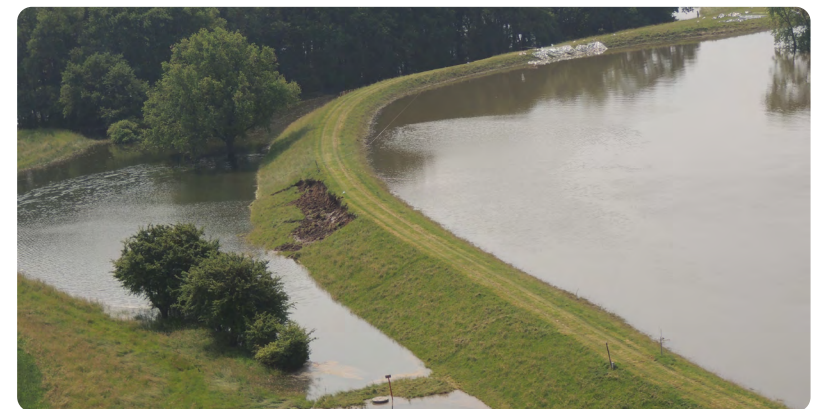
Figure 1: Macro-instability in Saxony-Anhalt (Germany) without flooding. Photo from Jüpner et al. (2015).
