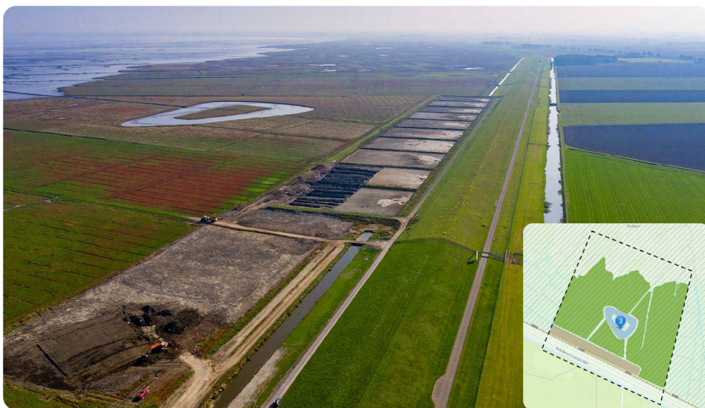
The Wide Green Dike section from above. Photo by the Regional Water Authority Hunze en Aa's.
