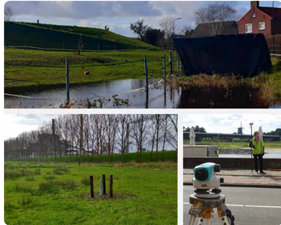
Figure 2: Top: Seepage through the dike and the subsoil (Photo by Waterschap Rivierenland). Bottom: Tube that is placed in the soil to measure the groundwater (Photo by Waterschap Brabantse Delta) and fieldwork for data collection (Photo by Bas van der Meulen).
