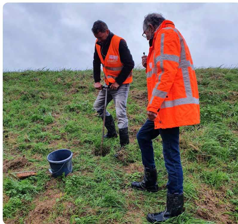
Figure 1: Soil drilling for analysis of the layers of a dike body. Photo by HWBP.
