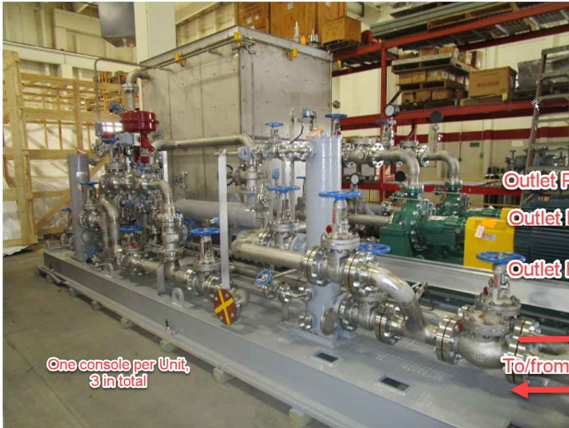
11-PK103 – Plan 54 Console – final inspection at Lube Power in Detroit area, May-2015
