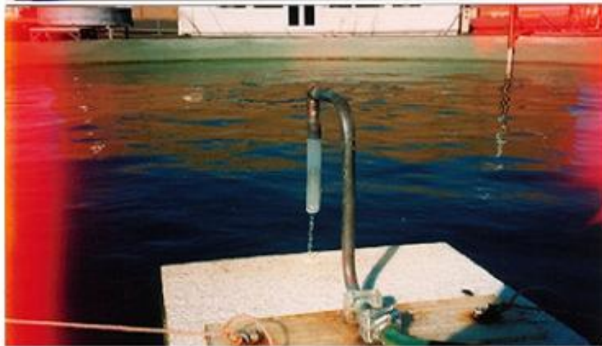
Fig. 4: Flushing arrangements at Magnesium chloride pond
