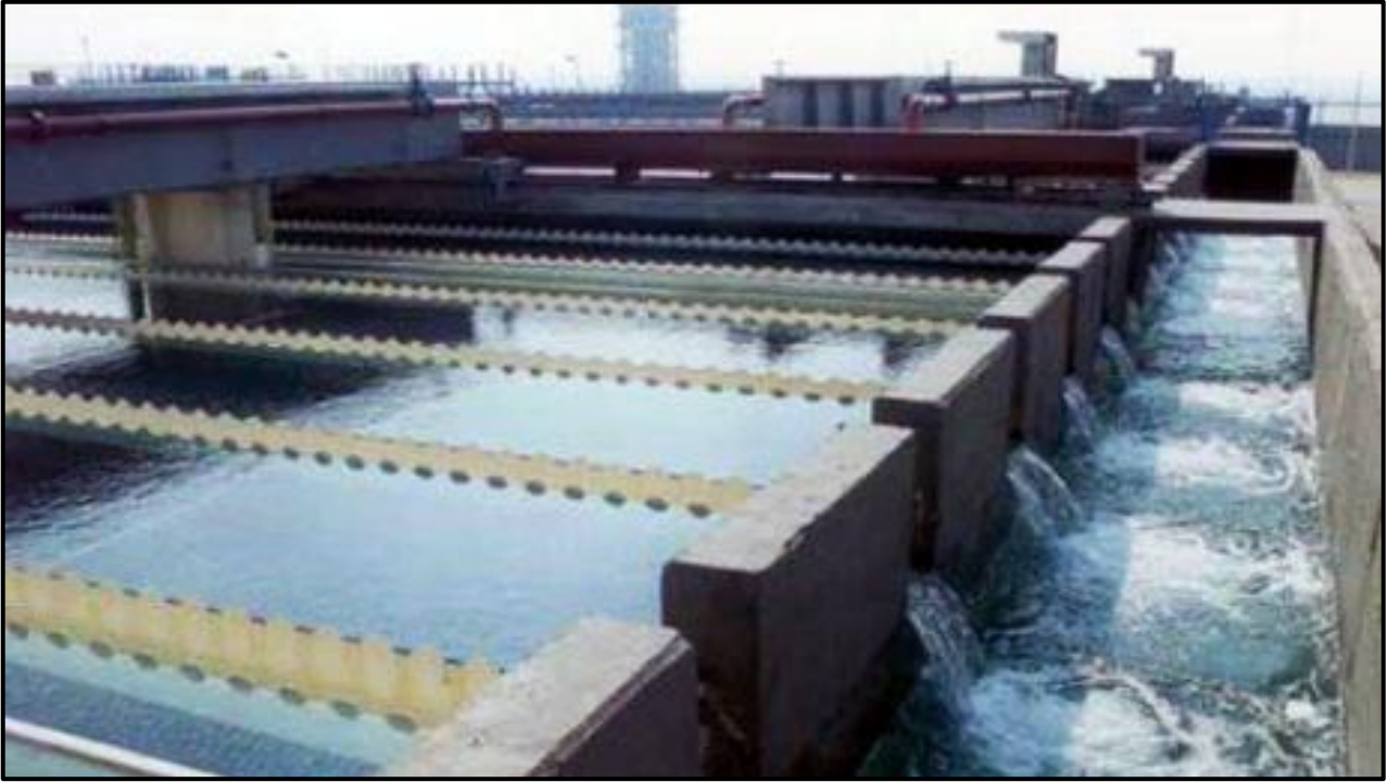
Water Treatment Plant in Egypt
