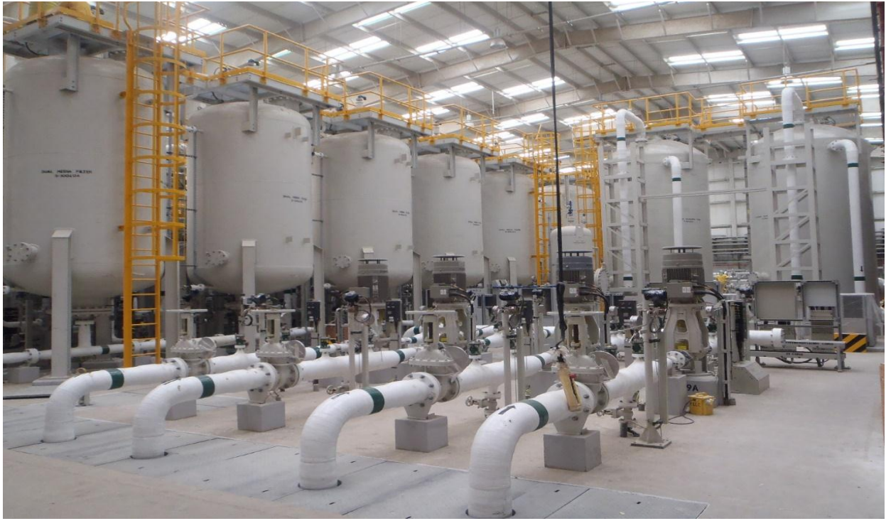
Qatar - Halul Island : R.O. Desalination Plant
