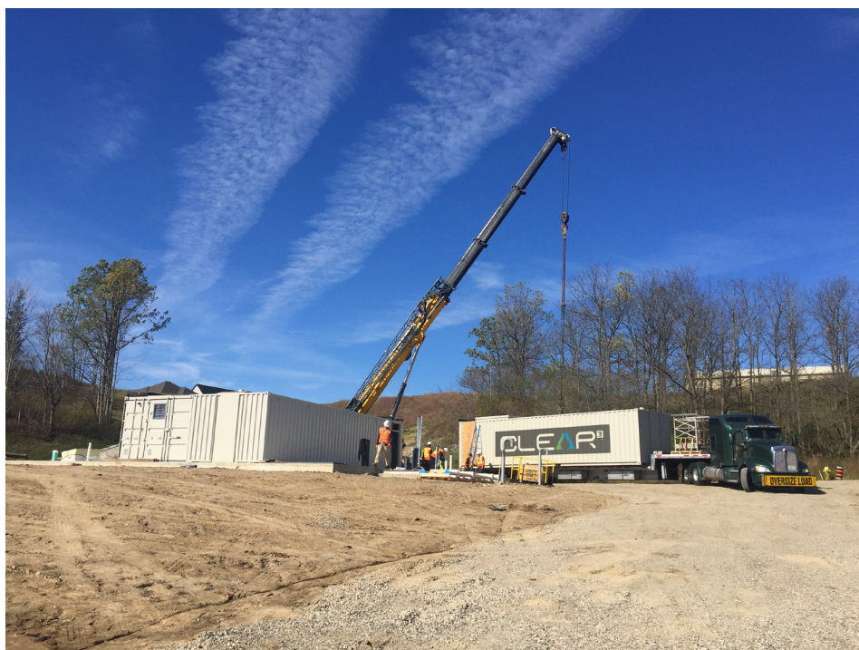
Figure 2. This Newterra (132,000 GPD) Clear3 MBR system was installed in one day for this new residential development in the small township of Southwold, Ontario, Canada. The system was designed with the option of being expandable to 317,000 GPD to accommodate the future expansion of new homes.
