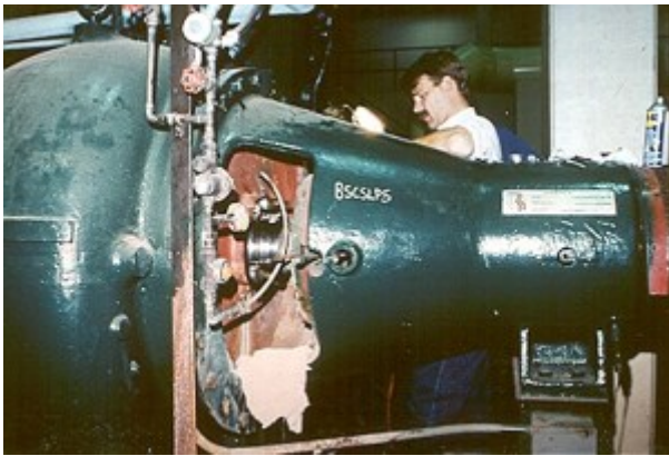
[ Large centrifugal waste water pump]
