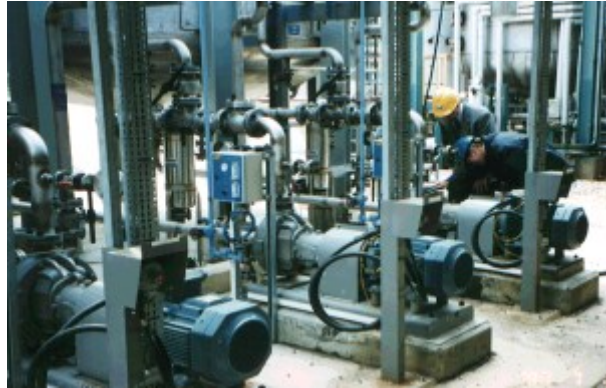
The simple gas barrier supply system can be seen in this photograph. This supplies clean, dry gas to the non-contacting seals.
