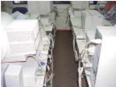
Neatly organised wiring for easy cleaning
