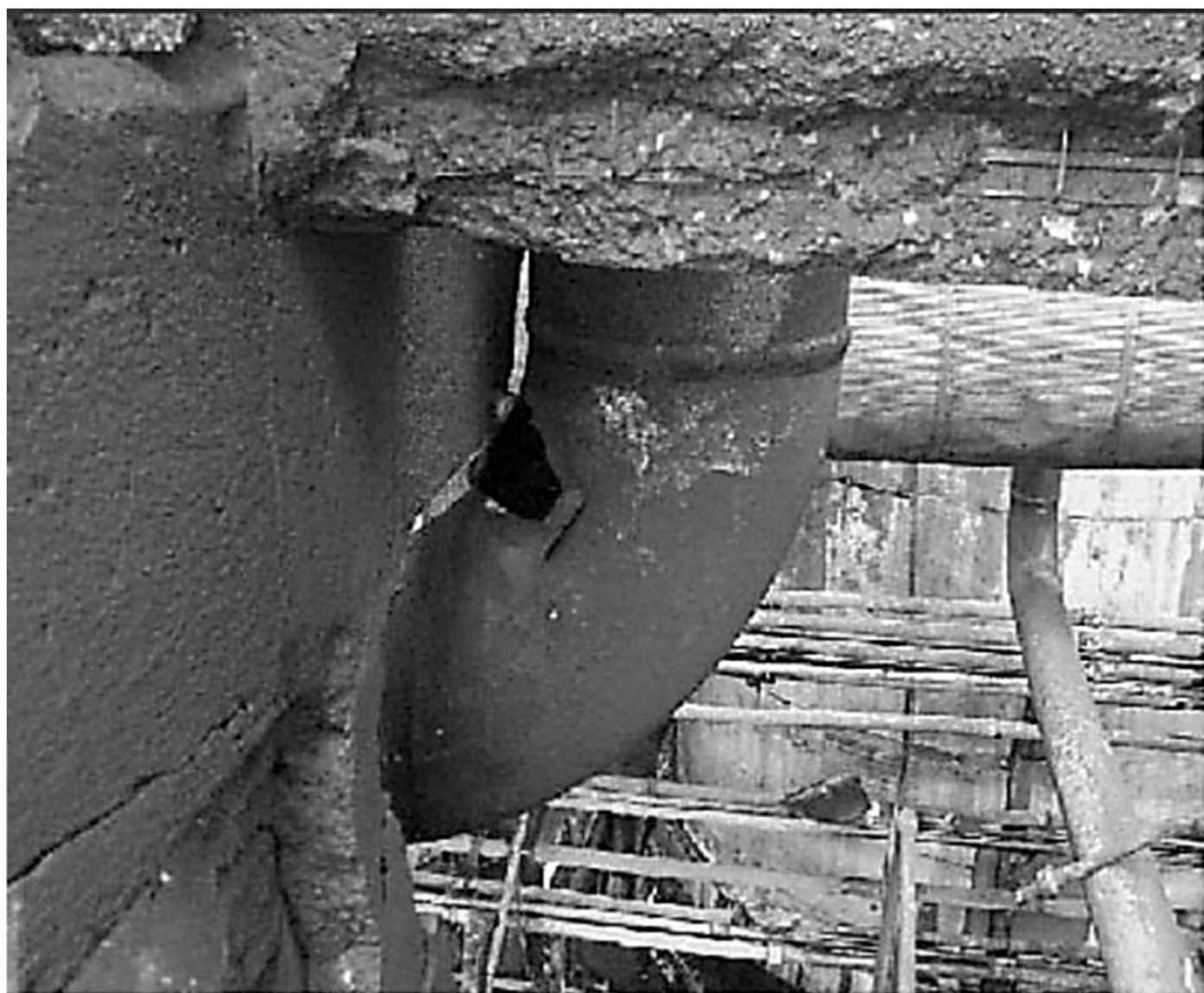
Figure 4-120 – Sulfidation failure of piping elbow.
