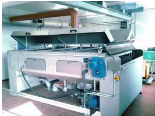
WWTP Bramsche / Germany
