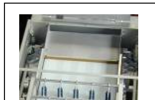
Sludge intake on same width as belt
