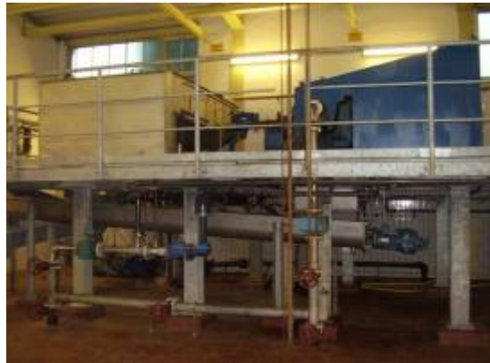
WWTP Löningen / Germany
