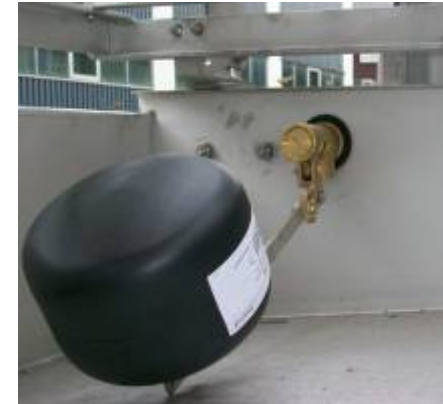
Float valve to control additional process water
