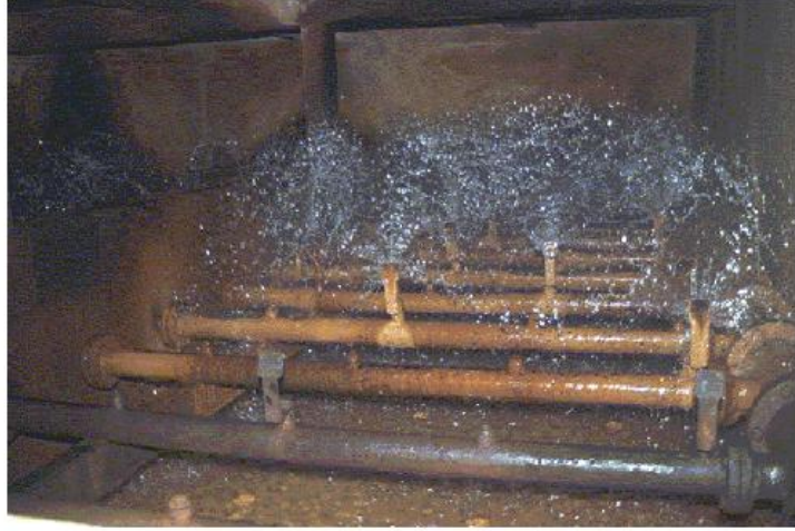
Figure 4 - Aeration above limestone filter
