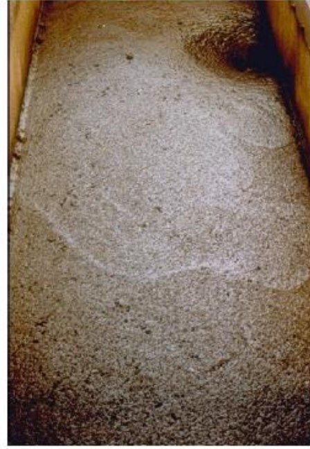
Figure 20 - Result of a poorly designed filter bottom
